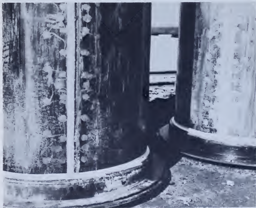
Figure 162.—Forms for cast pipe. If tight gaskets are not used in form joints, gates in inside forms and joints with base rings should be sealed with 2-inch cloth tape that will adhere firmly throughout the placing operation. Paper tape is not fully satisfactory. PX-D-34610.
